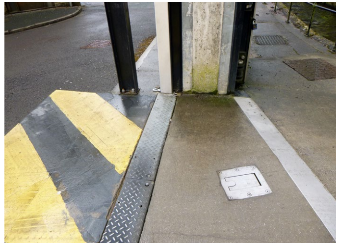
Previously installed steel access plates had deformed
