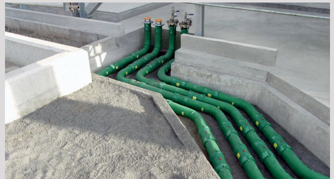
Ethanol Power Plant, Reunion Island
